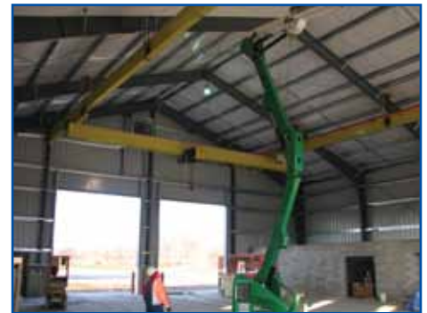
10 ton overhead crane installed in new shop
